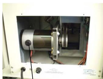
Two brush holders (Installed on the other side of this face shown in this photo)
